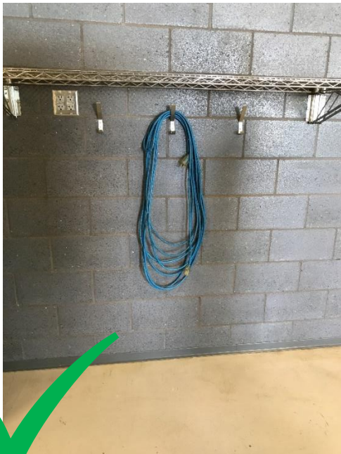
Acceptable when not in use, per MN State Fire Code 605.5
